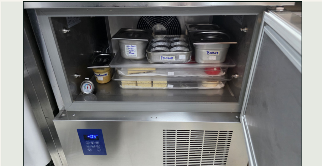
Blast chiller used as regular refrigeration. (Source p. 23)
